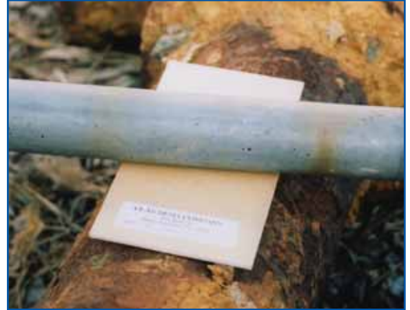
Prevent or correct underground contacts between mains.
